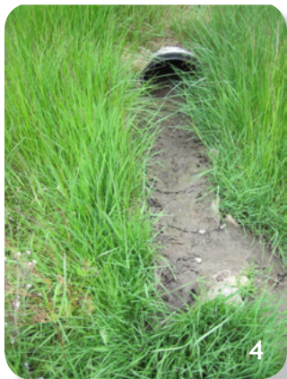
Photos 2 and 3. Examples of short-circuiting ponds. Photo 4. Pond with excessive sediment deposition.
