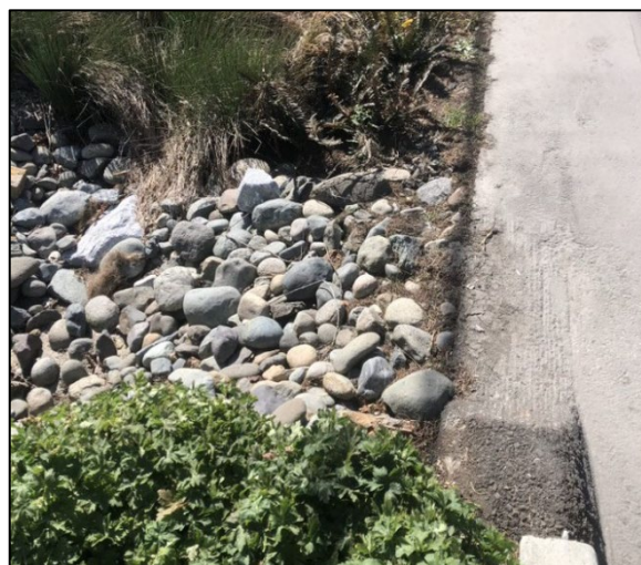
Figure A-14. Observable Sediment at Road Edge.
