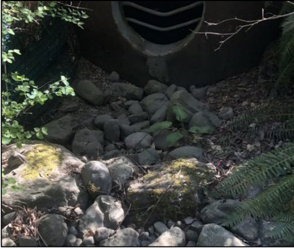
Figure A-7. Relatively Clean Inlet Area on 110th Cascade.
