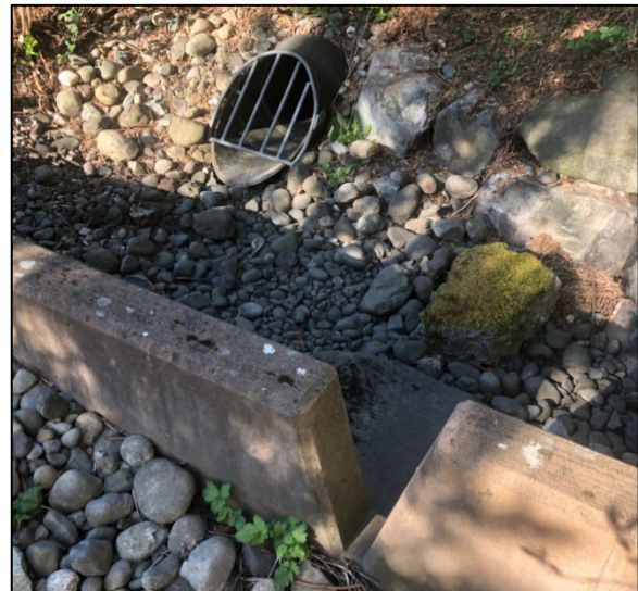
Figure A-2. Last Cell of First Block Below Greenwood Avenue North on 107th Cascade.
