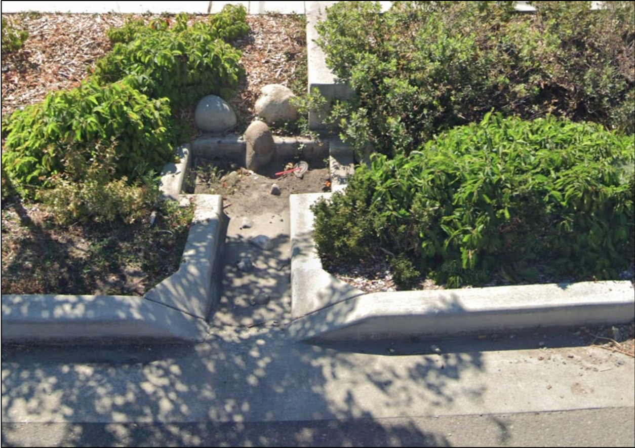
Figure A-18. T117 Inlet with Sediment via Google Street View (August 2019).
