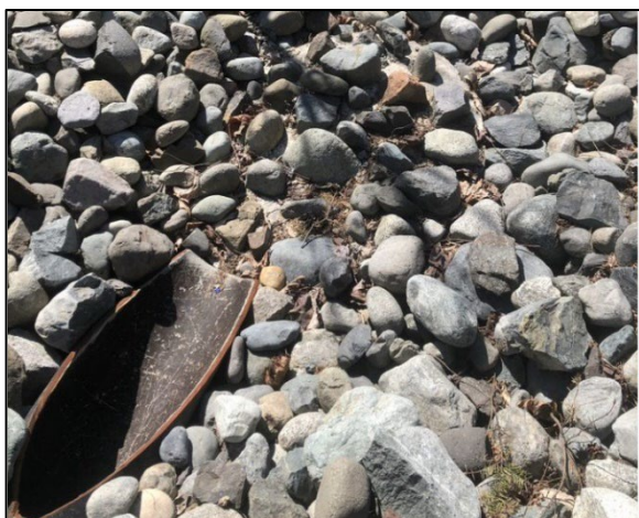
Figure A-13. Cell Inlet at Northeast 135th and 30th Avenue Northeast.
