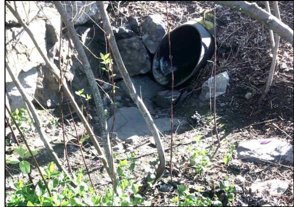
Figure A-1. Entrance to First Cell Below Greenwood Avenue North on 107th Cascade.
