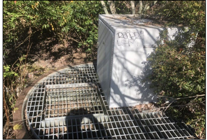
Figure A-8. Remnant Monitoring Equipment Enclosure Between Greenwood Avenue North and Palatine Avenue North Along 110th Cascade.
