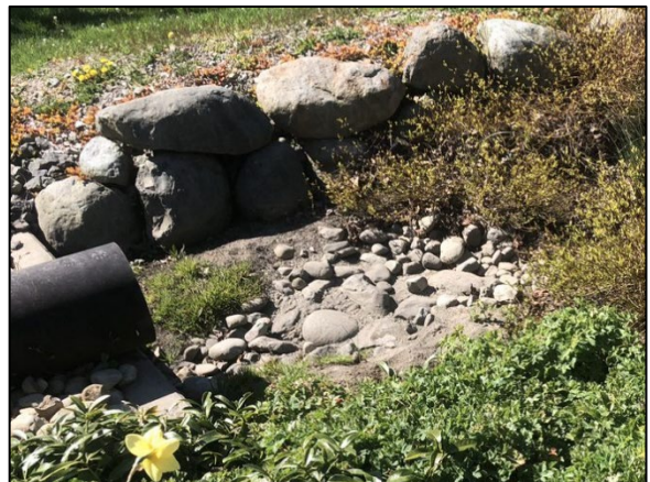
Figure A-12. Inlet with the Most Accumulated Sediment (sediment appears to be primarily sand).
