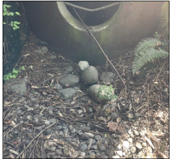
Figure A-6. Some Accumulated Sediment and Scouring near an Inlet on 110th Cascade.
